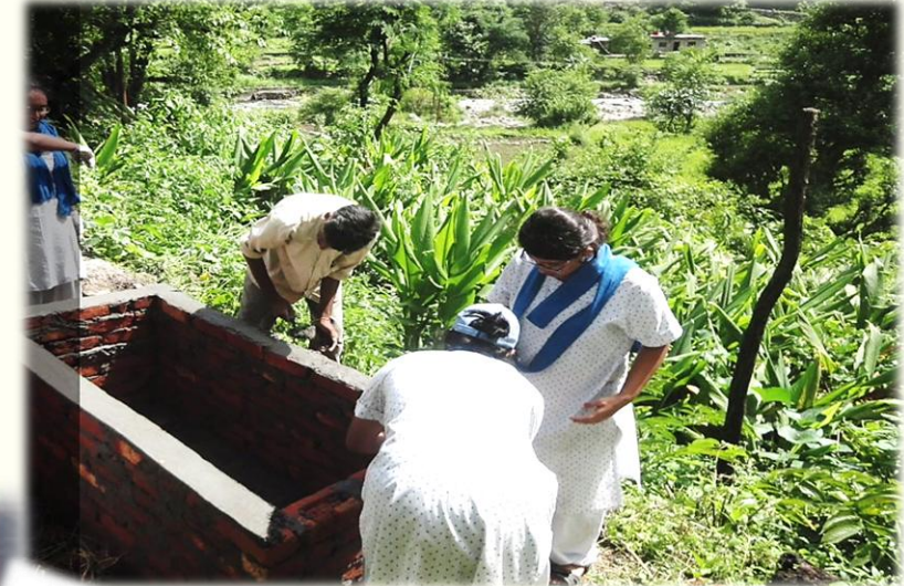
Biogas Digester Plant
